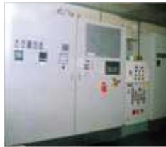
Control System for VP
